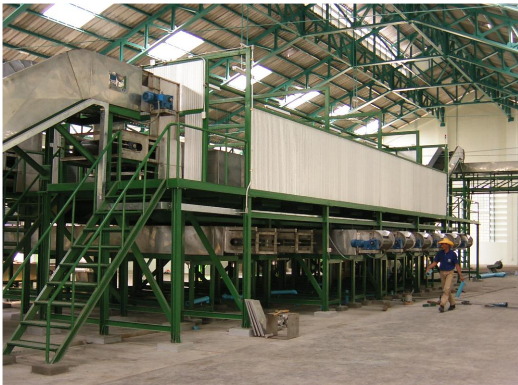
SORTING MEZZANINE AND RECYCLE CONVEYER
